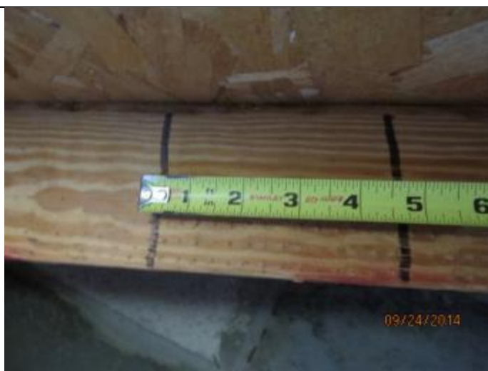
PHOTO 6 – Roof Deck Attachment Spacing
