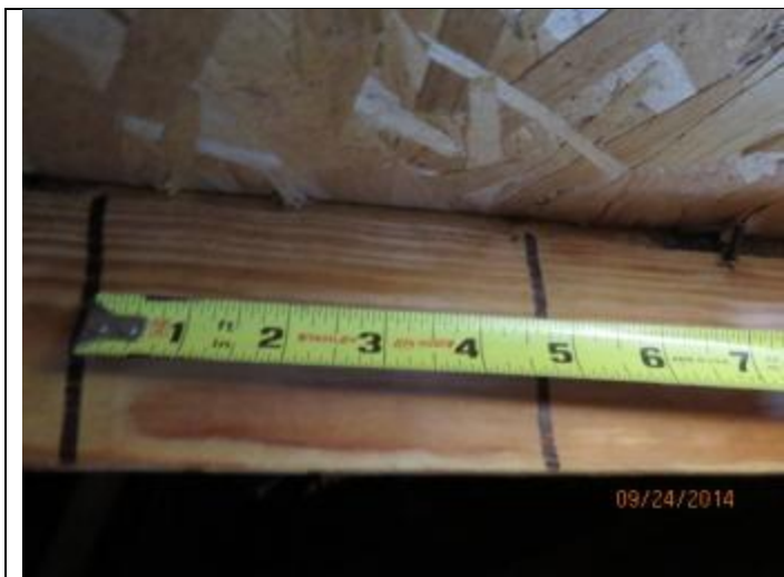
PHOTO 7 – Roof Deck Attachment Spacing
