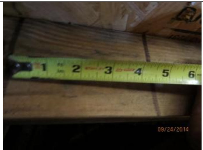
PHOTO 6 – Roof Deck Attachment Spacing
