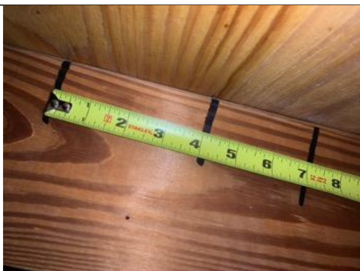
PHOTO 6 – Roof Deck Attachment Spacing
